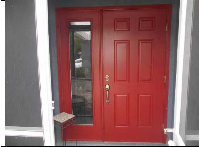
ENTRY DOOR – GLAZING NOT PROTECTED
