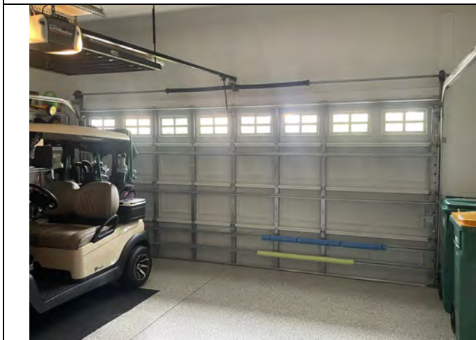
GARAGE DOOR – NO LABEL. 5 BRACKETS 8 FASTENERS.
