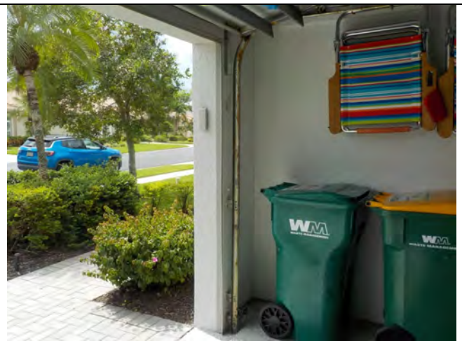
GARAGE DOOR – NO LABEL. 5 BRACKETS 8 FASTENERS.
